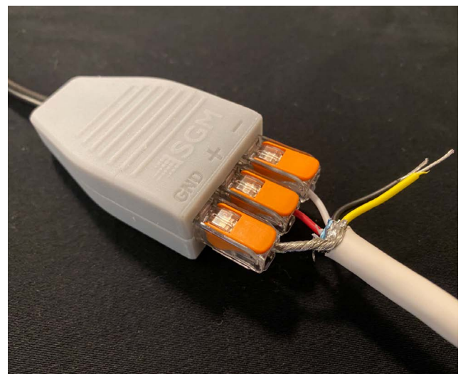
Figure 9: Connecting data to USB up-loader cable for POI fixtures
